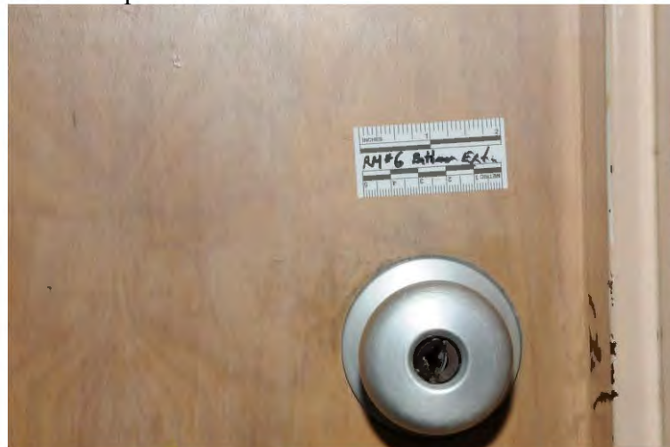
132 Example classroom restroom door lock - exterior
