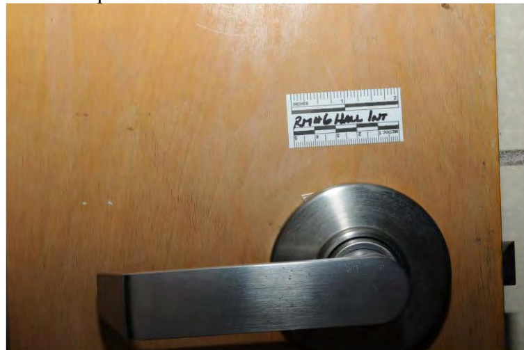
137 Example classroom door lock – interior
